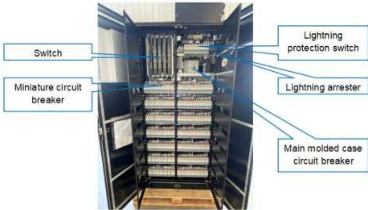
Figure 5-8 Internal view of distribution cabinet
