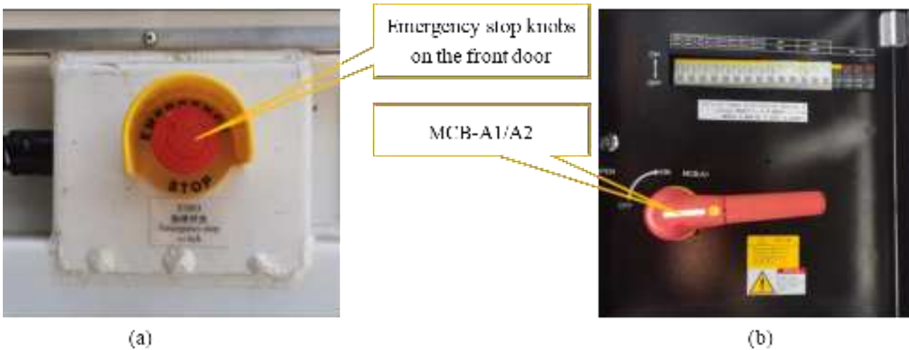
Figure 7.1 (a) Emergency stop knobs on the front door (b) Location of MCB-A1/A2.
