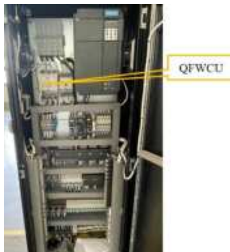
Figure 7.22 Internal view of the main switch of the main control cabinet.
